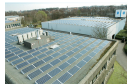
Solar panels installed on the roof of the company building
